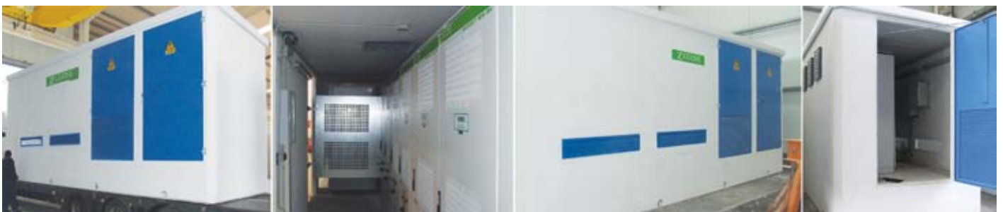
Sunzet Power Station
